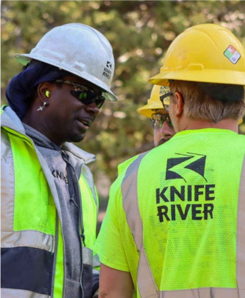
One of our Central Oregon asphalt paving crews conducts a job-hazard analysis prior to beginning work on a residential street.
